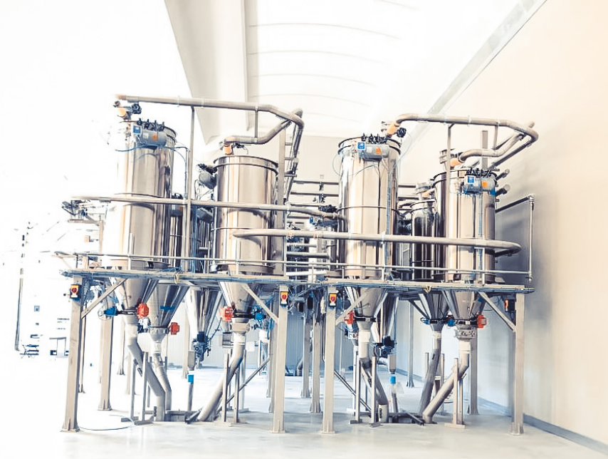
Two dosing points with four hoppers each
