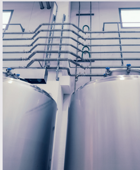
Automatic loading with heated pipeline
