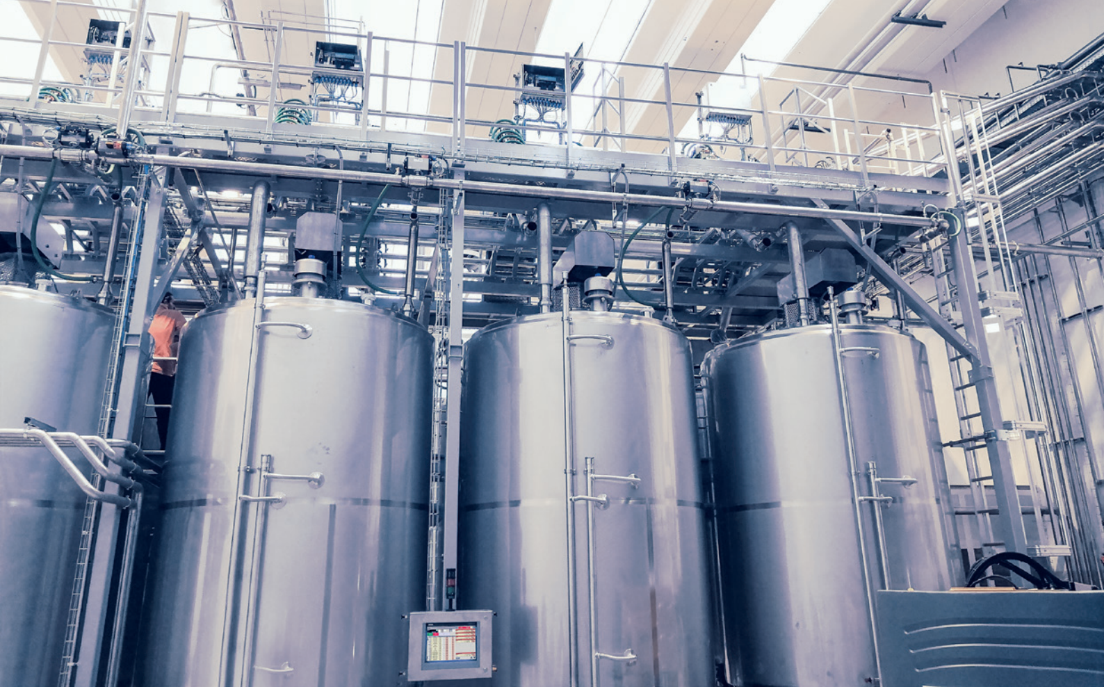
Liquid preparation and dosing tanks with HMI
