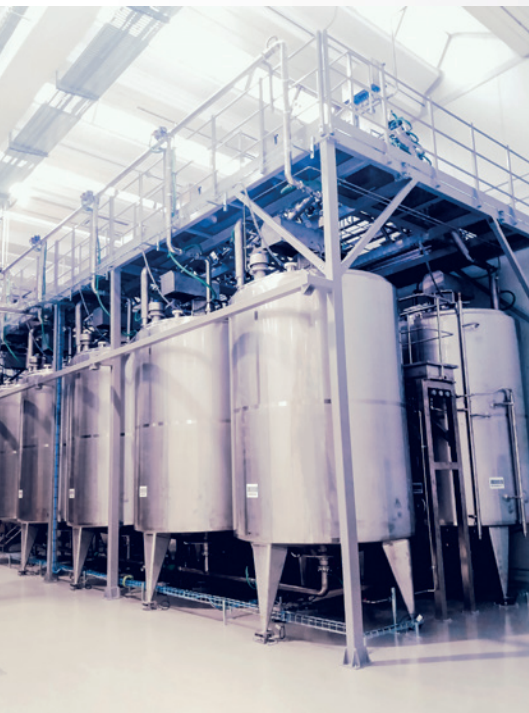
Double jacketed tank group with maintenance platform
