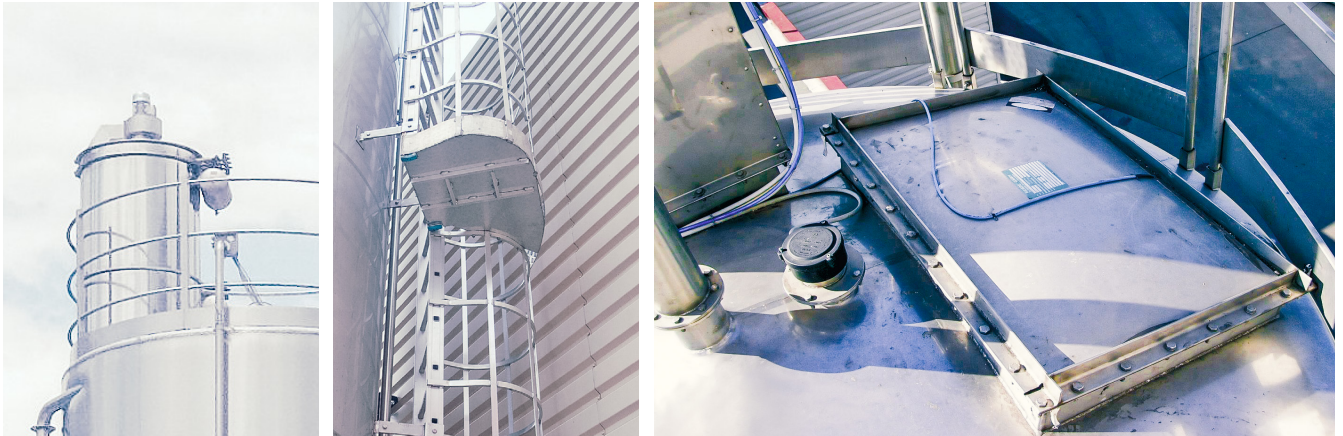
Powder recovering filters, ladder and bursting disk
