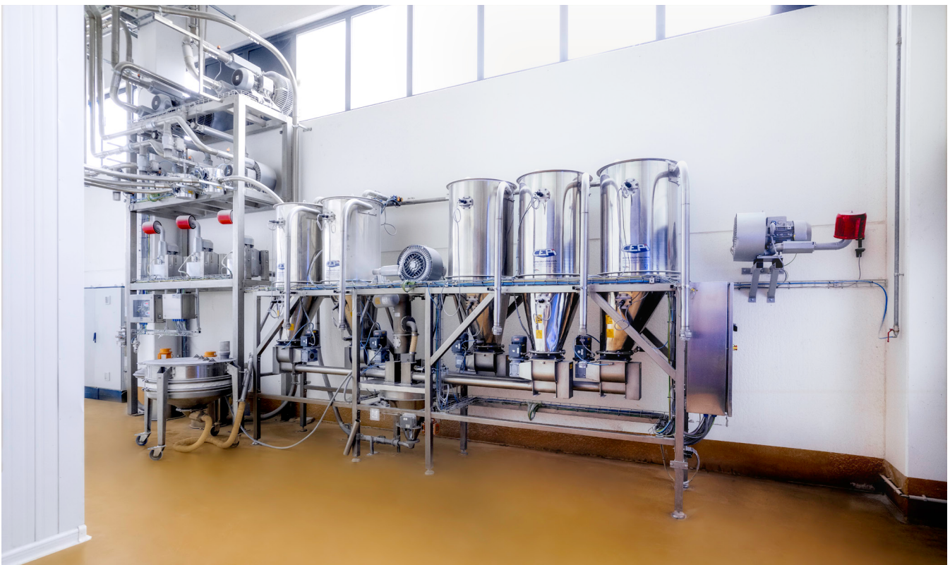
Microingredients station fed by dump station
