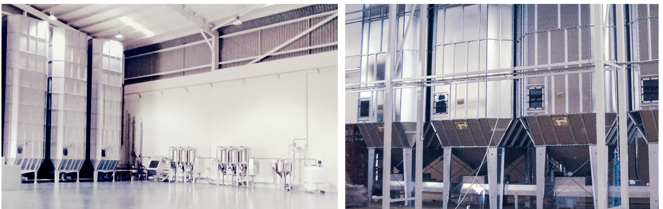
From left to right: installation with silbox silos, microingredients stations and invert sugar system; silos for cous cous
